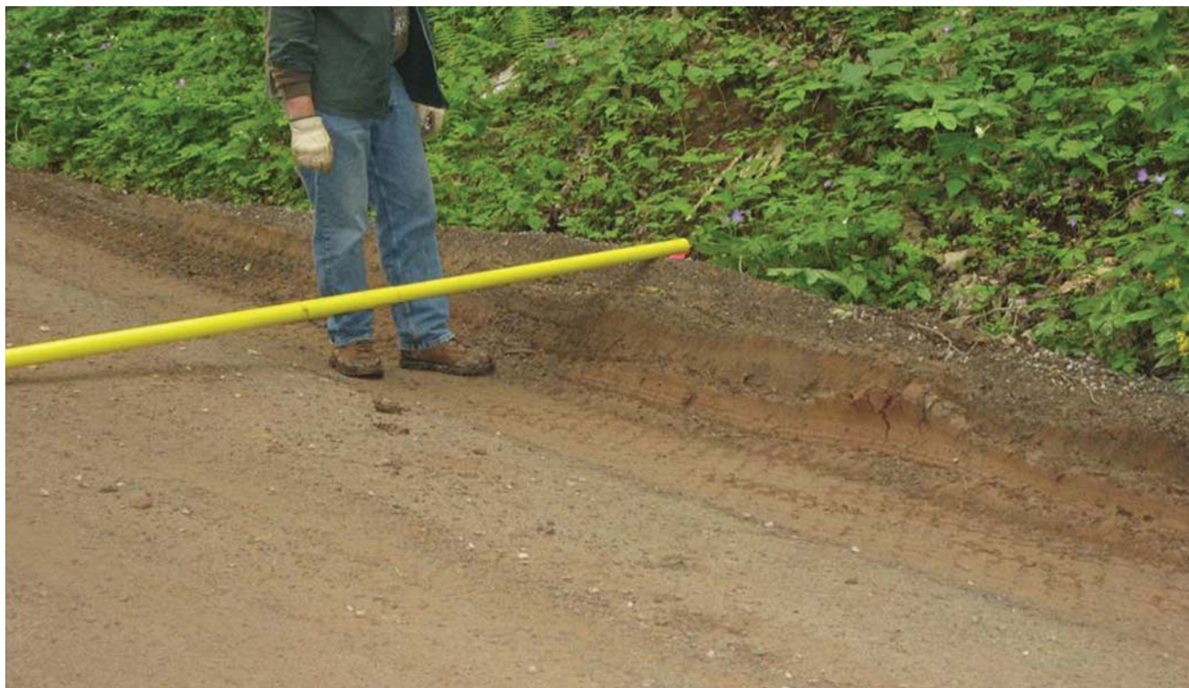
Figure 3. —Damage to road surface and roadside ditch on the Fernow Experimental Forest from gas well construction and drilling equipment. Note that the drainage ditch has been obliterated. Photo taken May 22, 2008. Photo by U.S. Forest Service.
